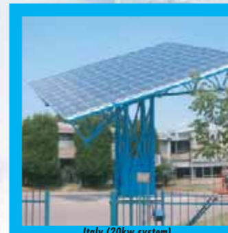
Italy (20kw system)
